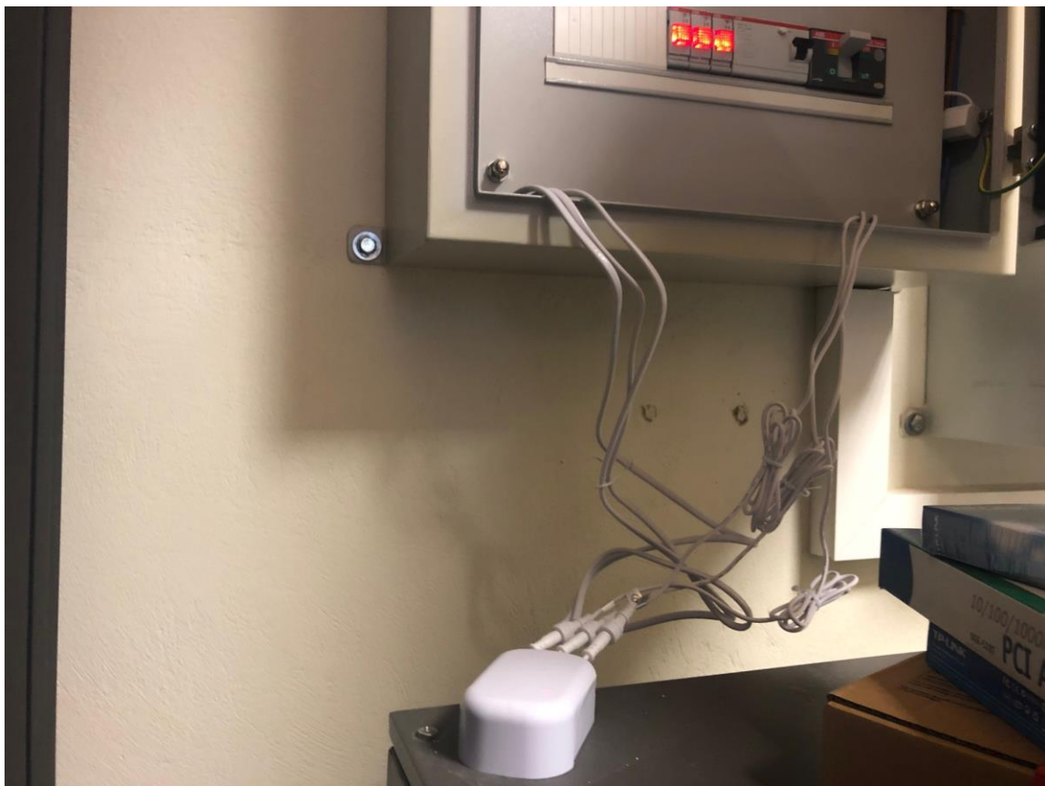
Figure 1: An indicative smart meter connected to the central fuse box
